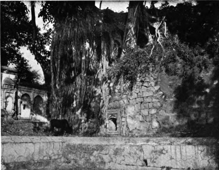
BANYAN ROOTLETS DESTROYING BUILDING, MAHOBA.
